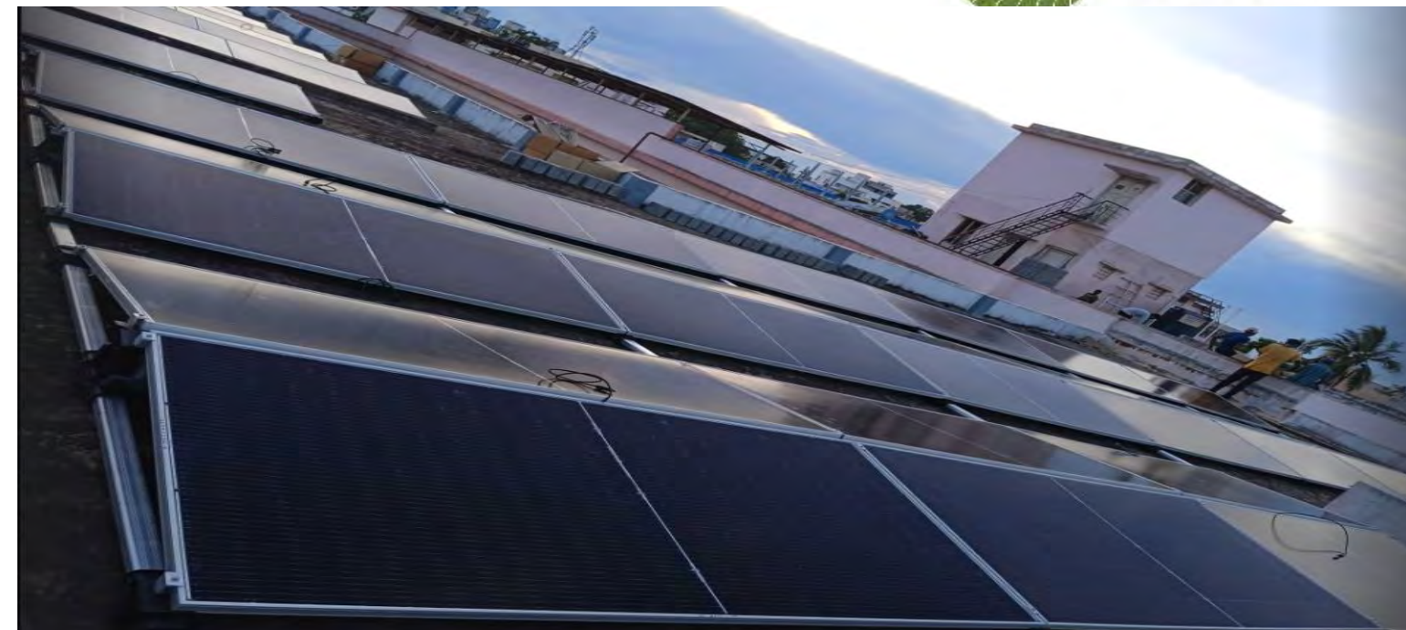
ST JOSEPH HOSPITAL -100 kWp
