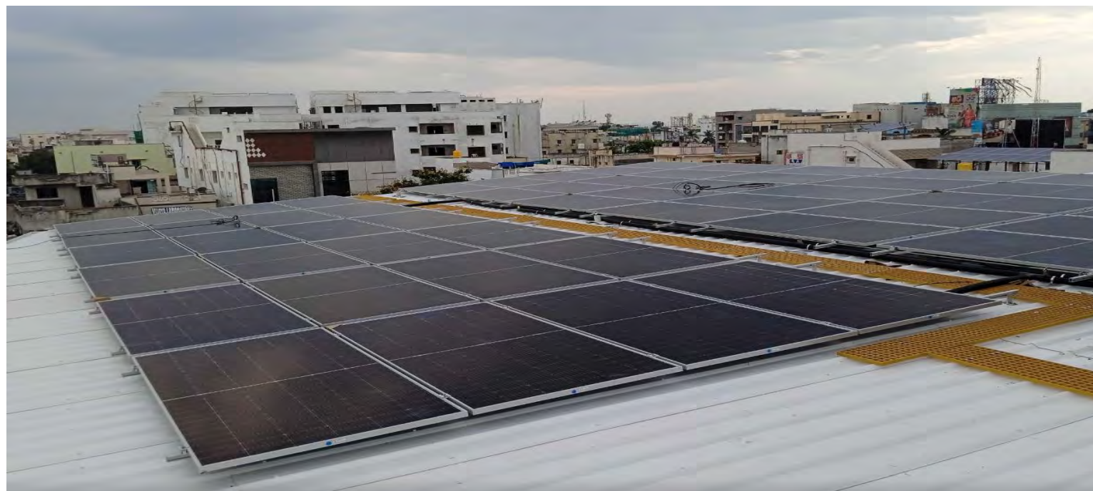
PEOPLES POLYCLINIC -100 kWp
