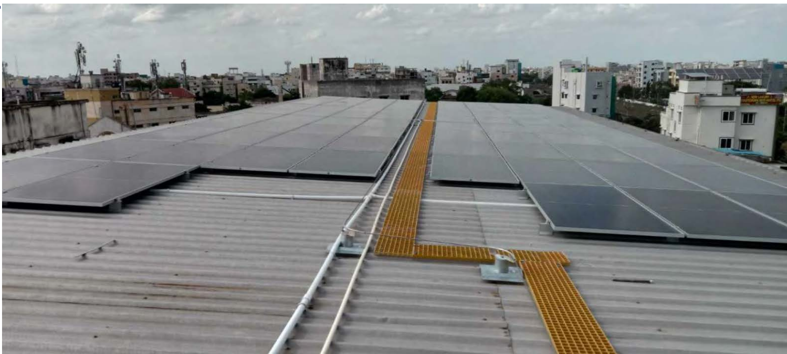
JAYABHARAT HOSPITAL – 50 kWp
