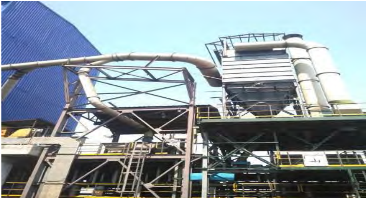
DUST EXTRACTION SYSTEM AT TRANSFER POINTS
